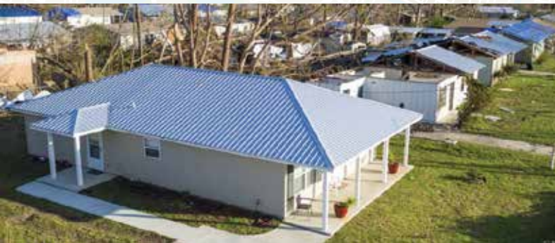
Built to the Fortified Gold standard by Habitat for Humanity, this home was undamaged by Hurricane Michael (2018).
