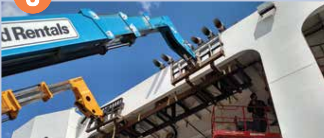
Two boom lifts are used to raise the wide curtain assembly into position.
